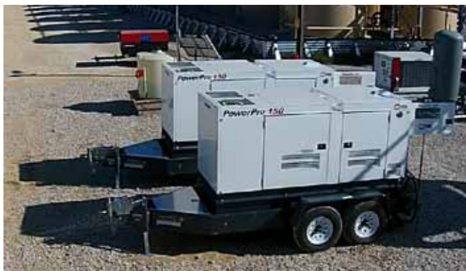
Oil and Gas — Production support power
